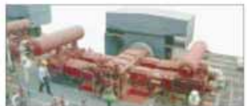
Two 5,500 horsepower HHE-VL hydrogen make-up units in a typical outdoor refinery application.
