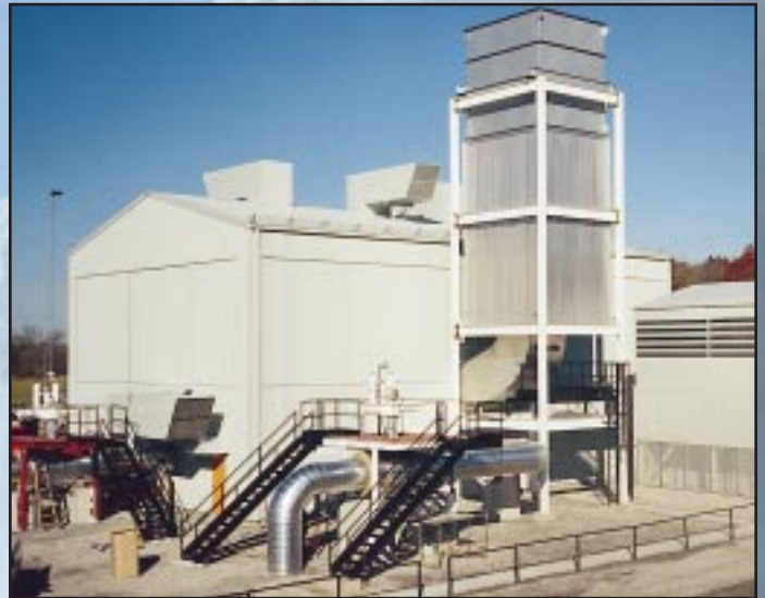
TransCanada Pipelines' Station 211C is located in Beamsville, Ontario, approximately 40 kilometers west of Niagara Falls.
